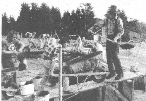
CEMENT HAULING — Forty-five people from the Seattle, Kent, Olympia and Tacoma, Wash., area moved 80 tons of cement in four hours to repair a swimming pool wall on Tanglewood Island, site of the Northwest Summer Camp. From left: Jeff Hermanson, Mike Skyles and Jim McConnell. (See "Church Activities," this page.)
